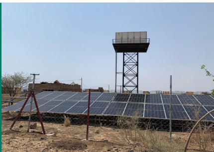
Solar panels at a water point
